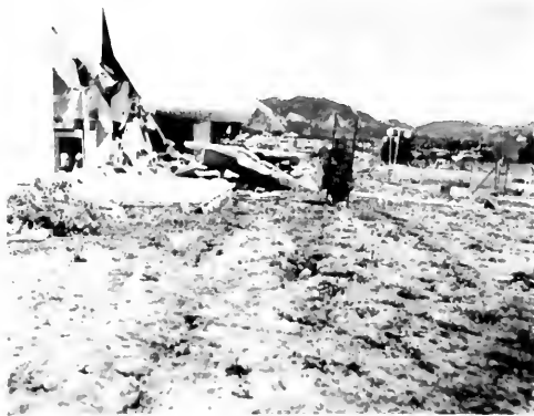
Photo 7. View east at southwest corner of Olive View Hospital main building; ground cracks formed as a result of spreading out and bowing up of fill to south of building, probably in response to movement of fill beneath building during shaking and collapse of south stairwell (barely visible). Photo by James E. Kahle.
